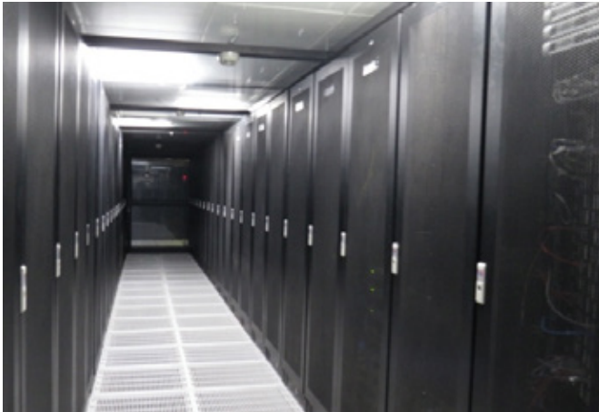
RailTel Data Center at Gurugram
