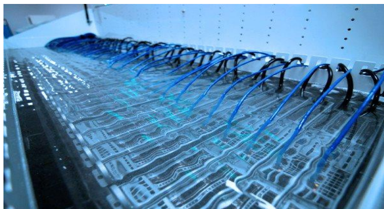
DATA Centre Cooling
