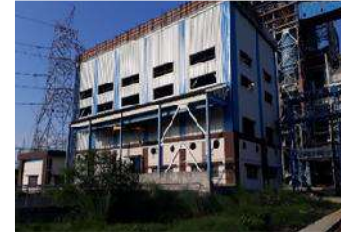
1X500MW, FGUTTP, CIVIL, STRUCTURAL AND ARCHITECTURAL WORK FOR BTP, BOP & CHP, UNCHAHAR, NBPPL
