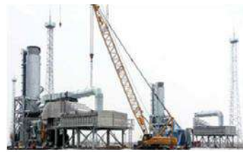
35 MW GT POWER PLANT, KAZAKSTHAN
