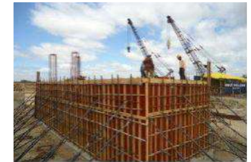
1X110 MW, CIVIL AND STRUCTURAL WORKS ,R&M OF MAIN PLANT, BATHINDA, BHEL
