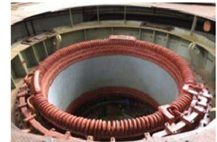
NEWLY REWOUND 30MW HYDRO GENERATOR AT UMIAM STG-III HYDRO PROJECT
