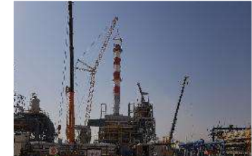
1519 MW FADHILI COMBINED HEAT AND POWER (CHP) PLANT KSA
