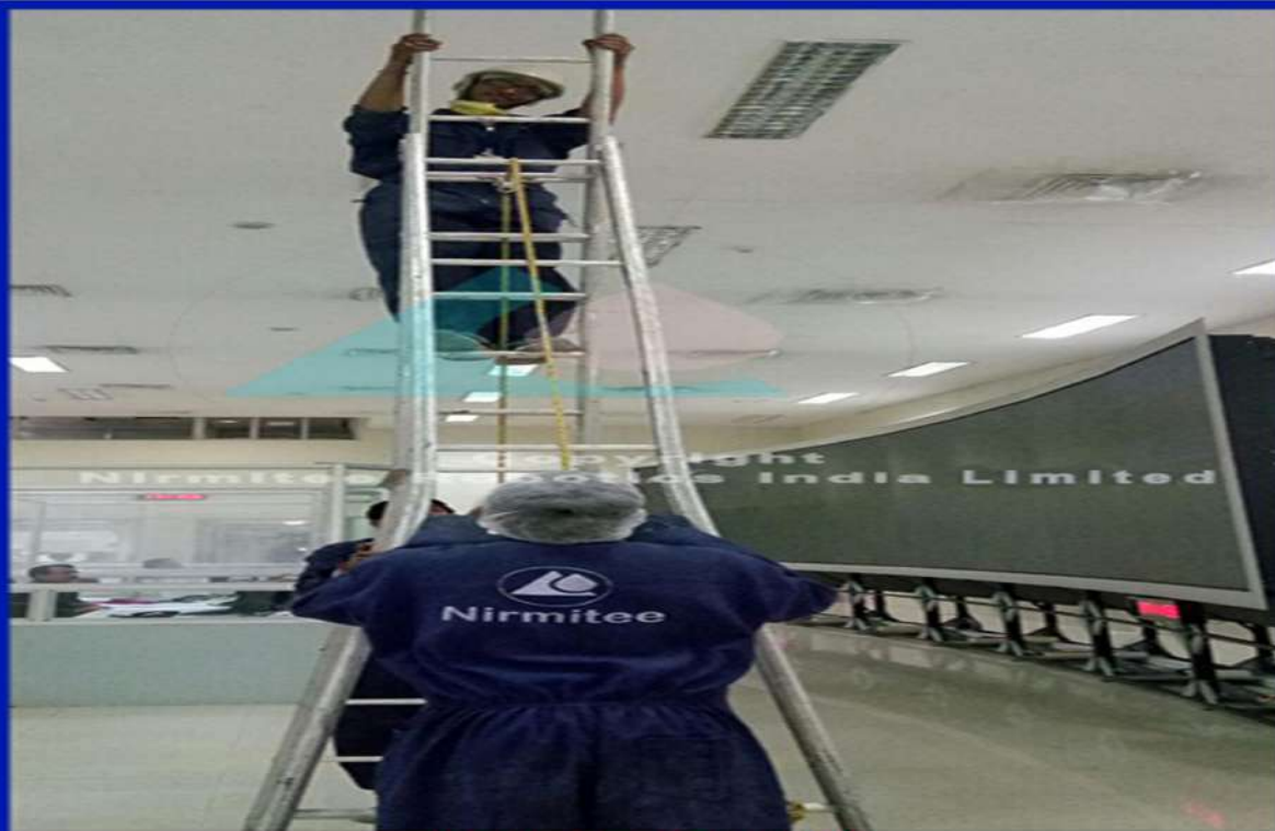
Our Speciality Critical Server and Projection Rooms
