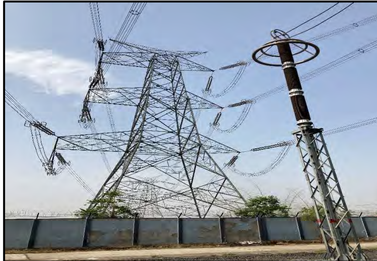
765 kV D/C Vindhyachal Pooling Station- Jabalpur Pooling Station line entrance at POWERGRID Jabalpur Substation
