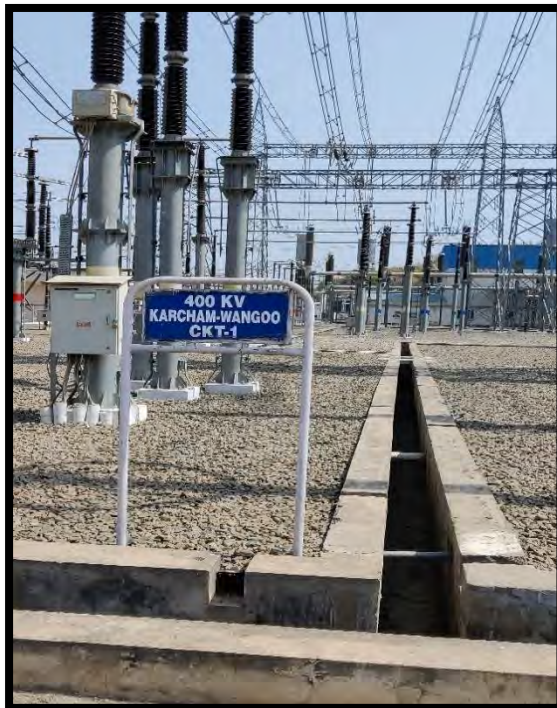
400 kV KARCHAM WANGTOO line bay
