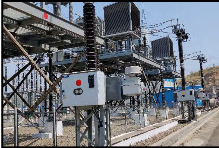
Fixed Series Capacitor
