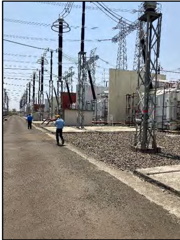
Inter Connected Transformer (ICT) – 7 x 500 MVA
