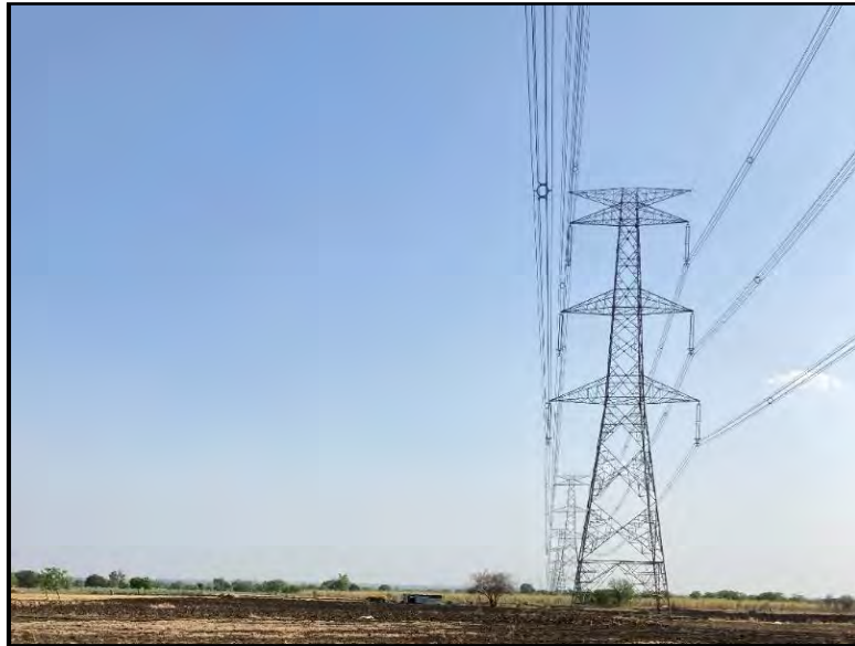
Transmission Line - 765 kV Parli (New) – Solapur Line
