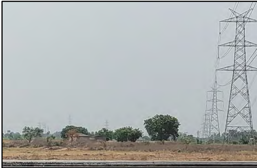
400 kV Transmission Line
