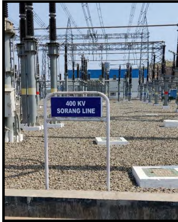
400 kV Sorang Line bay
