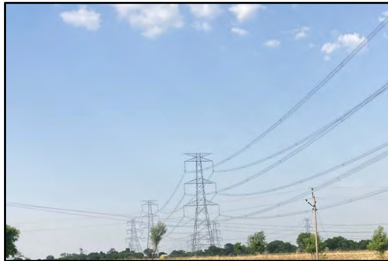
Transmission Line – Gadarwara to Warora – 765 kV
