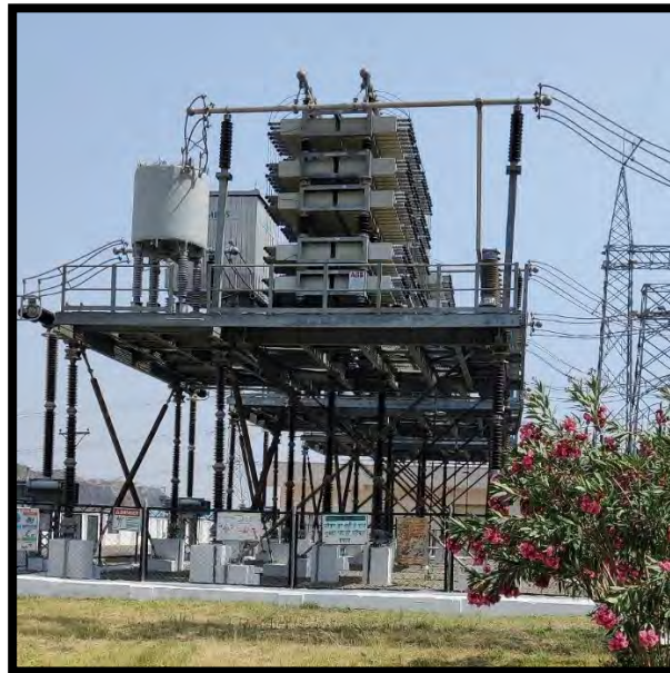
Fixed Series Capacitor
