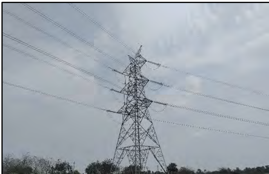
Angle Tower of 400 kV Transmission Line
