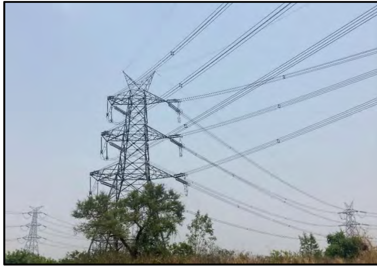
Transmission Line – LILO of both circuits of Wardha - Parli (PG) 400 kV D/C line at Warora* Pooling Station (Quad)
