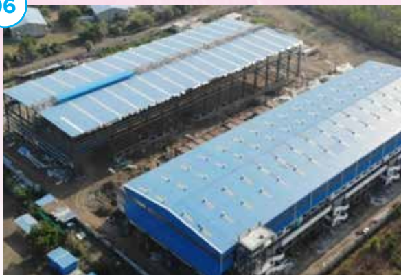
Location: Plot No. G-108, BUTIBORI MIDC, NAGPUR (M.S.), - 441108 INDIA (Factory Under Construction)
