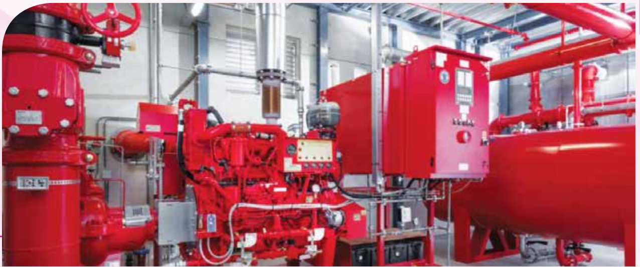
Fire Fighting & Hydrant Systems
