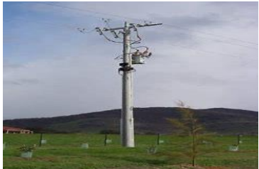
Power Distribution Poles
