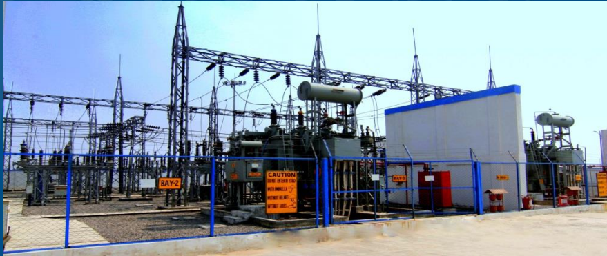
Tata Power - HT Substation
