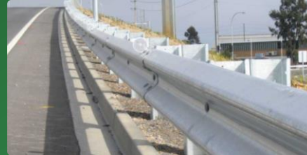
Metal Beam Crash Barrier
