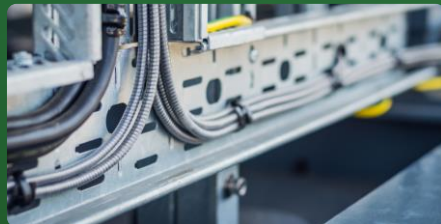
Cable Tray & Earthing Material
