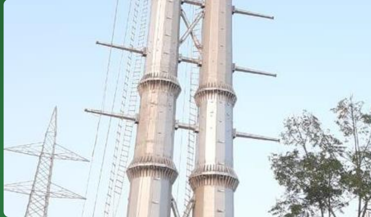
Transmission line Monopoles
