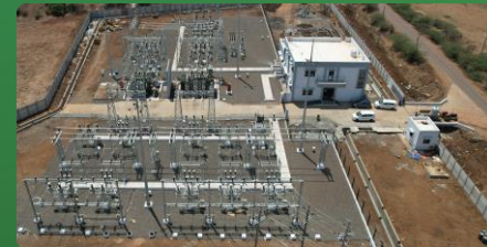
Pooling Sub-Station Development
