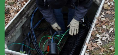
Optical Fiber Fault Rectification
