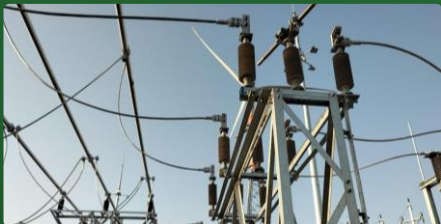
Isolator (HV Disconnectors)
