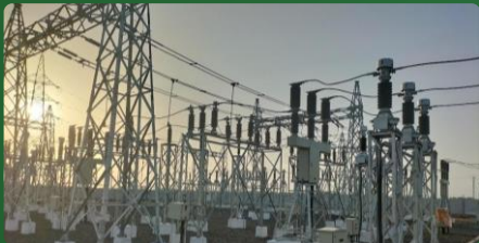
Sub-Station Equipment Structure
