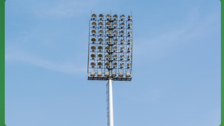
High Mast Poles & Lighting Poles
