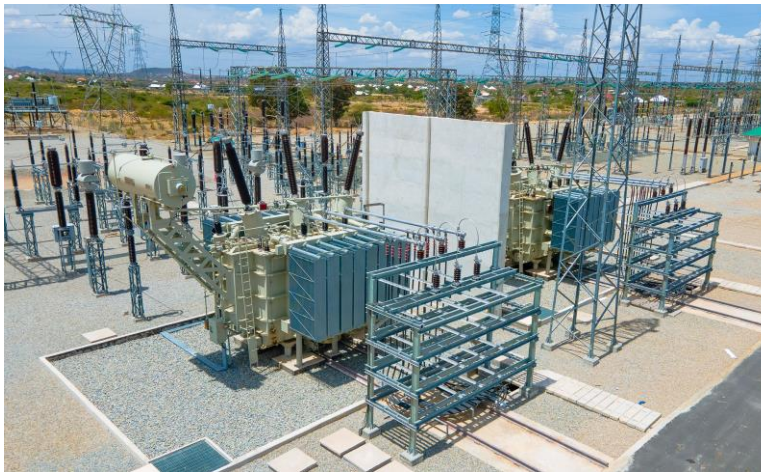
HVDC Converter Stations
