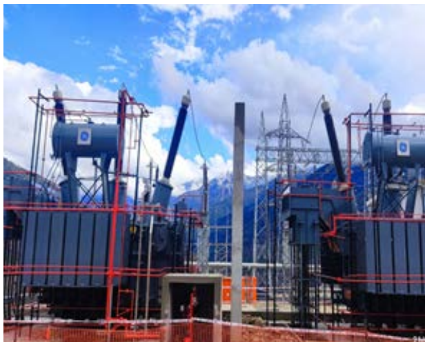
GE's first 220 kV Gas Insulated Substation in Bhutan for Bhutan Power Corporation
