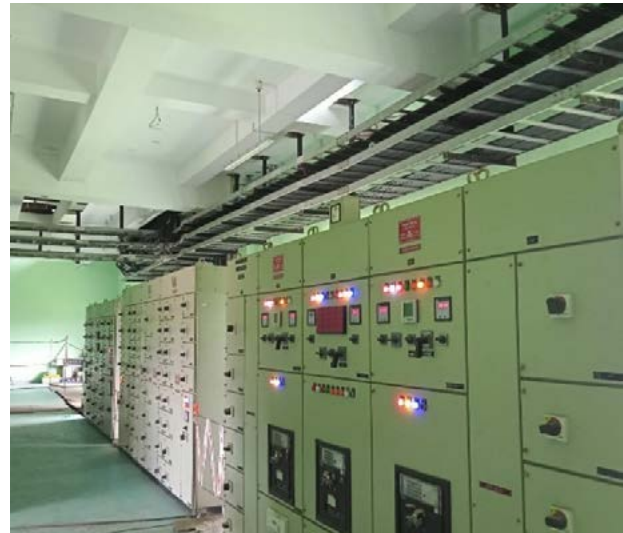
33KV GIS at Birlapur in West Bengal
