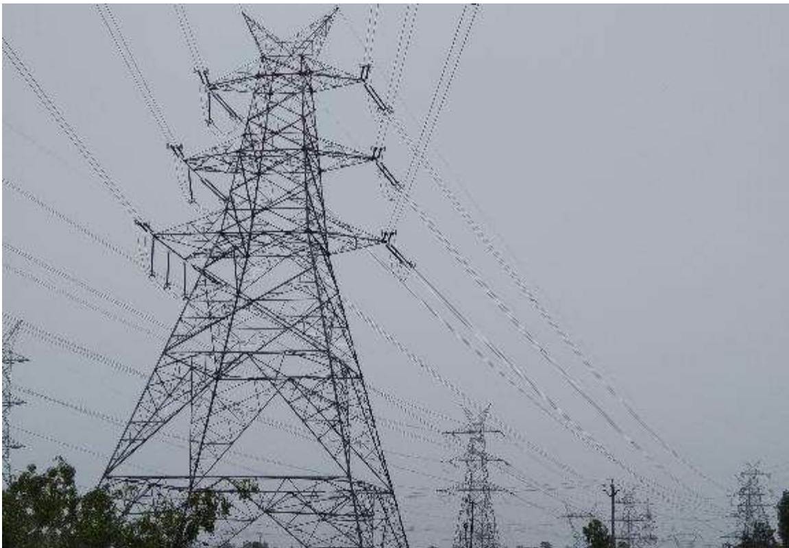
Jalandhar – Samba 400 kV D/C Powerline crossing
