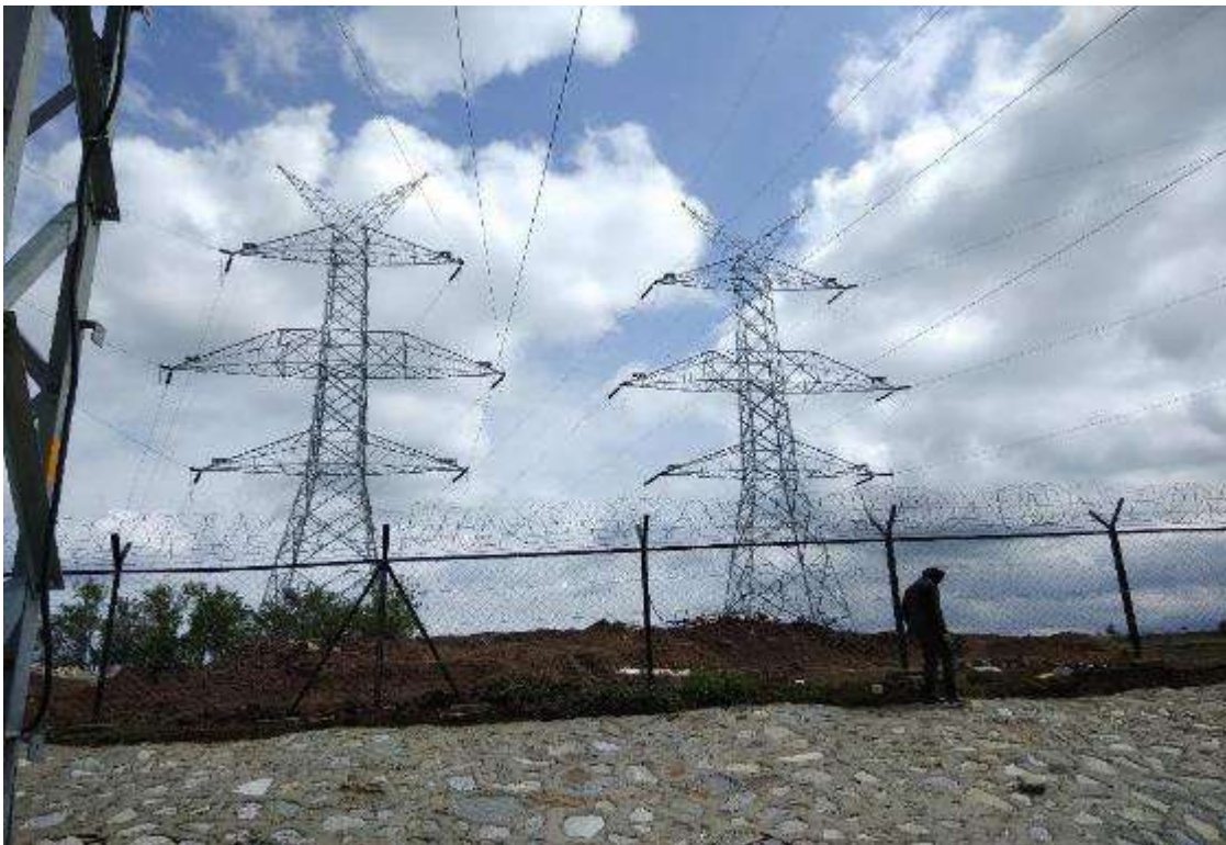
220 kV outgoing transmission lines
