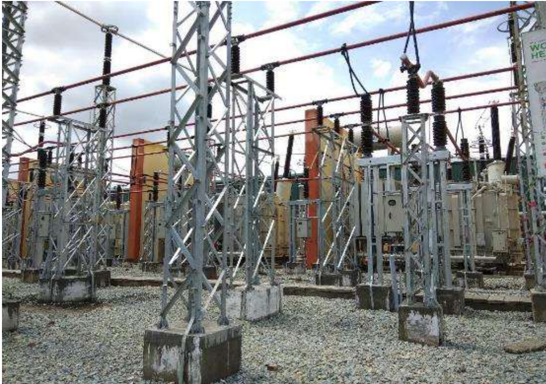
Inter – Connecting Sub – station yard
