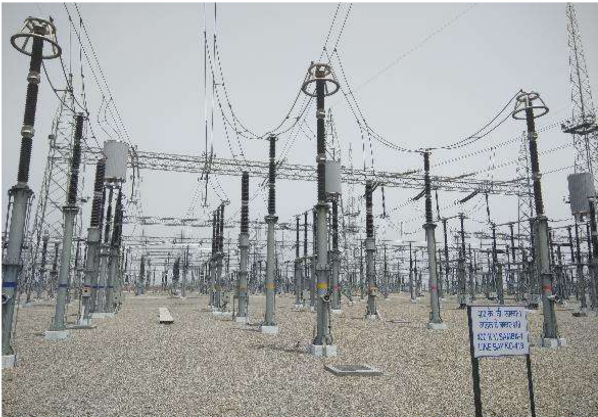
400/220 kV PGCIL Substation at Jalandhar Samba Line 1 Bay
