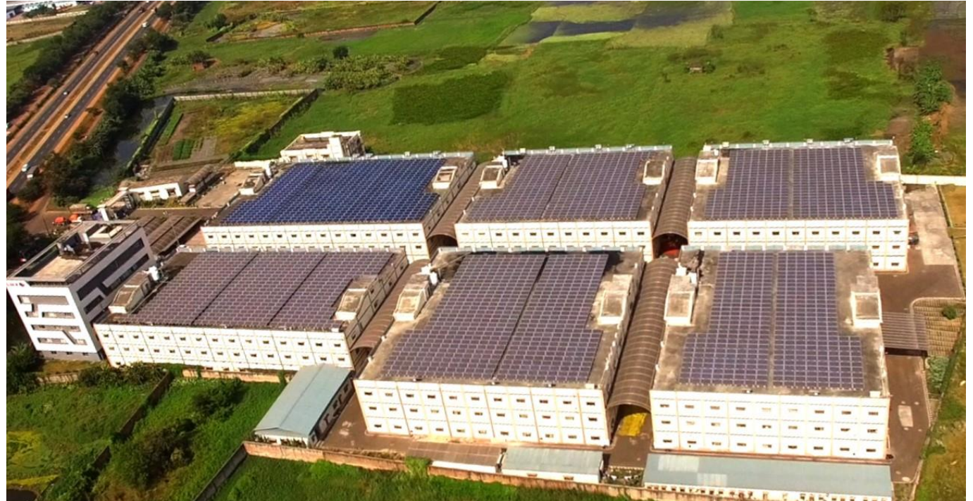
Rooftop solar power plant at Dankuni unit
