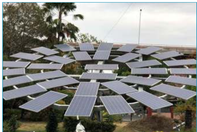
Solar tree installed at MOIL's Corporate Office
