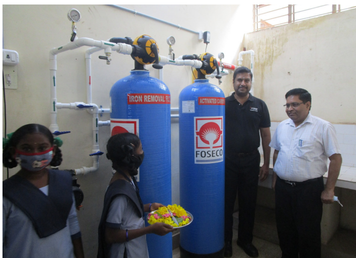
Water Treatment Plant in a School at Puducherry
