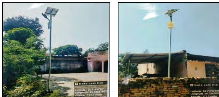
Solar lights at public places of Barabanki, Uttar Pradesh
