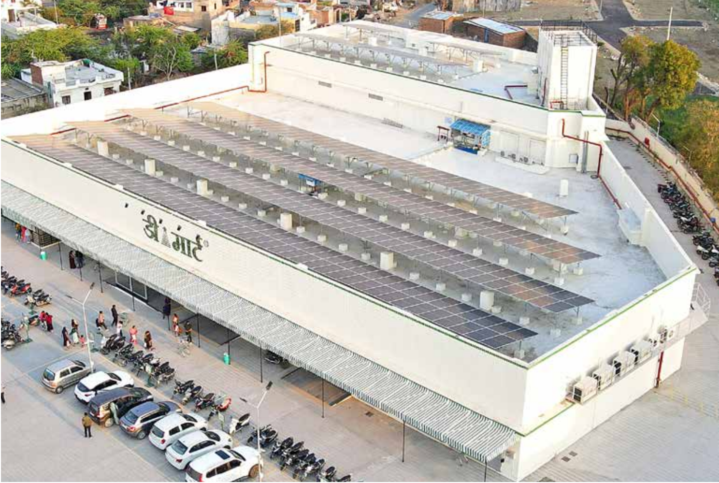
Rooftop Solar Panels
