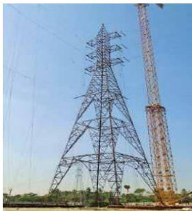
220kV Transmission Tower
