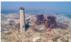
2X660 MW at Rampal, Maitree, Bangladesh-BIFPCL
