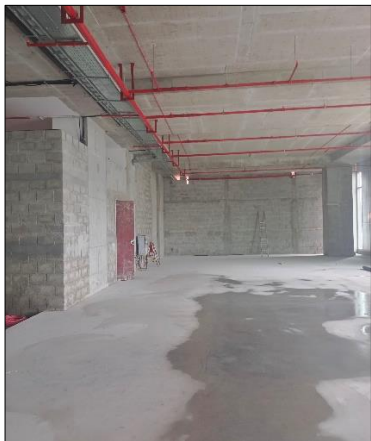
Internal View of the SP
