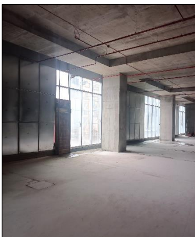
Internal View of the SP
