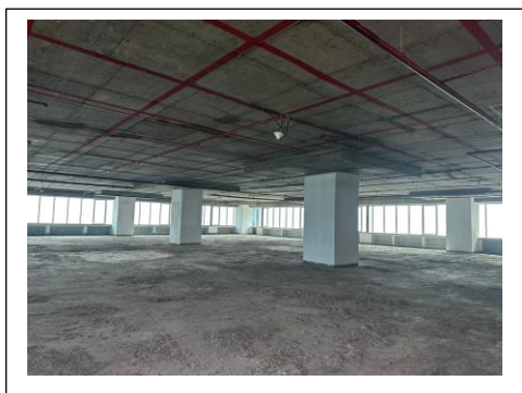
Internal view of the SP
