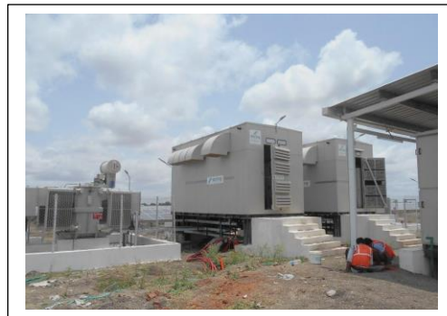
View of the solar power plant
