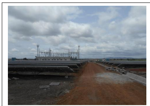
View of the solar power plant
