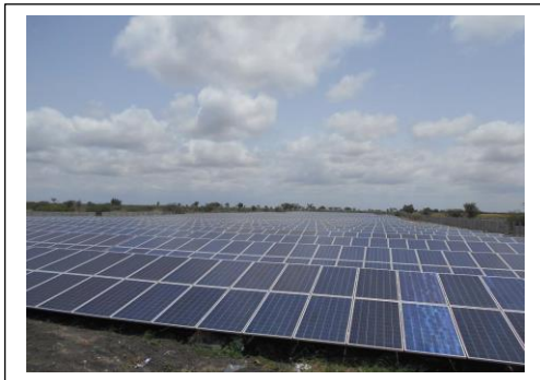
View of the solar power plant
