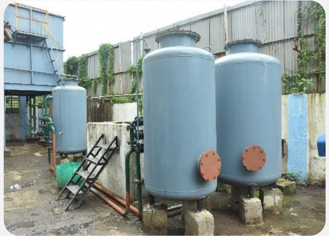
Effluent Treatment Plant
