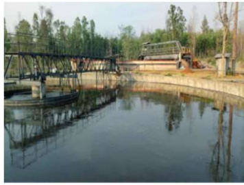
Secondary Clarifier - Pulp
