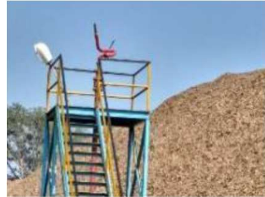
Fire Hydrant Point near chipper
