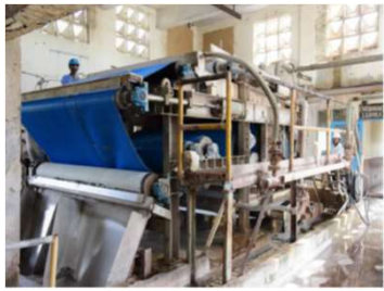
Sludge Handling - Paper
