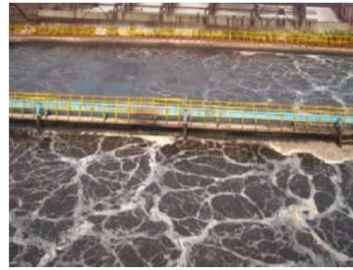
Diffused Aeration System
