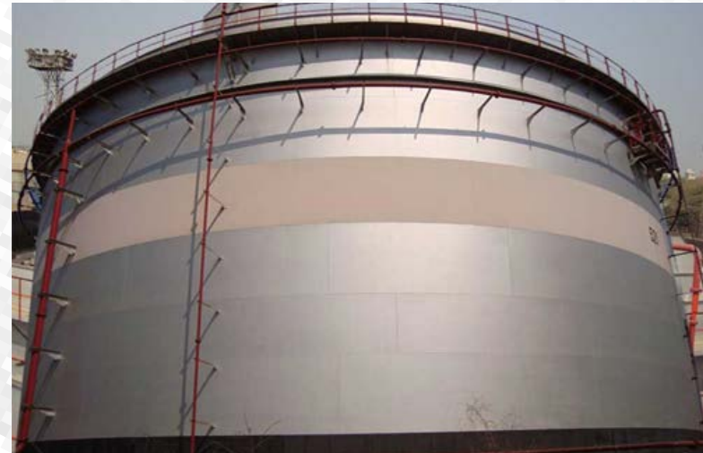
Floating Roof Tanks
