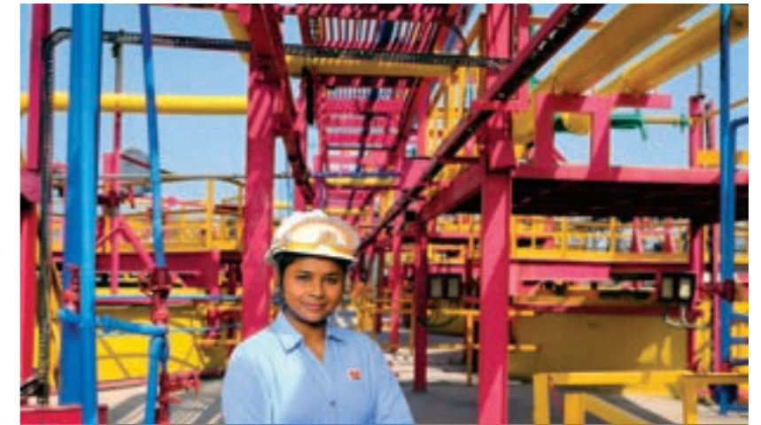
A view of our Renukoot refinery. Technology such as suspension calciner and slurry pumps (Geho) which were tried and tested a long time back, are now present in every refinery
