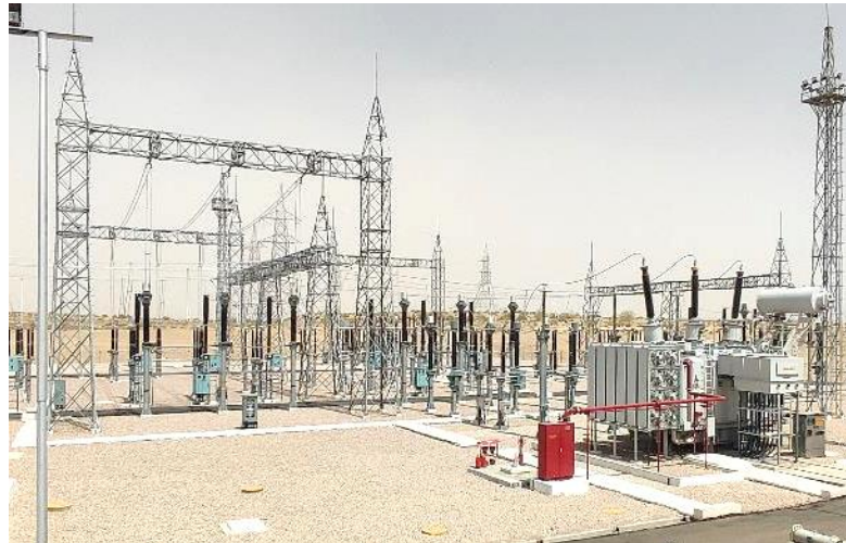
100 MW SECI Solar project, Banipura: Design, Engineering, Supply, Erection, Testing, Commissioning & Energizing of 220/33kV bay extension package
