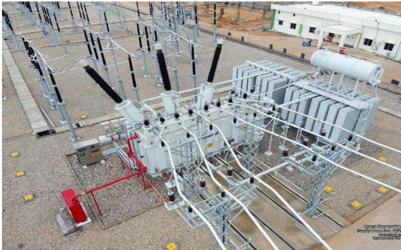
400/33 kV AIS S/s & 350 AC & 432 MW DC Solar Project, Bikaner: Design, Engineering, Procurement, Supply, Installation, Testing & Commissioning
