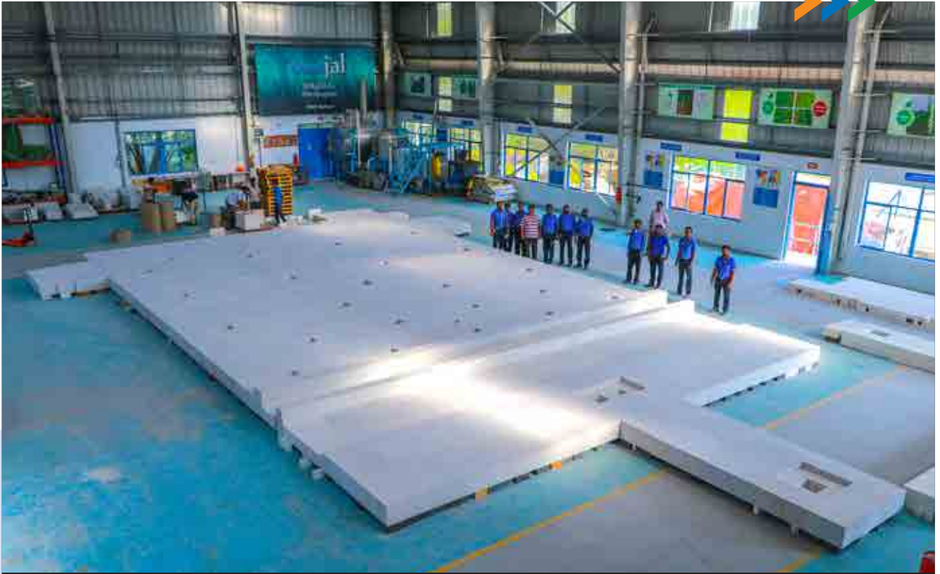
Execution team with bottom block assembly with 23 meter length X 14 meter width dimension
