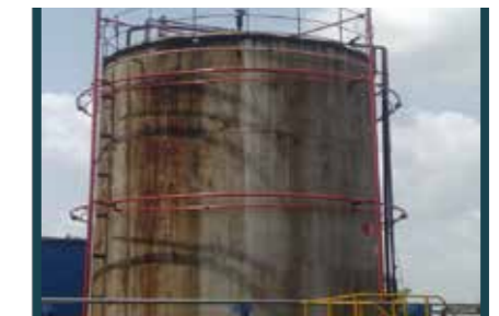
Sprinkler provision for methanol storage tank safety
