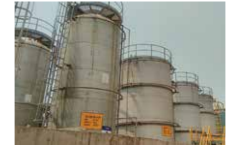
Sprinkler provision for Oleum storage tank
