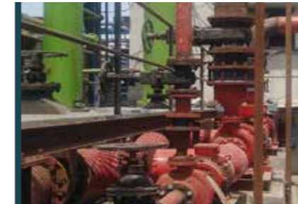
Fire hydrant capacity upgraded with 410 m3 pumping capacity
