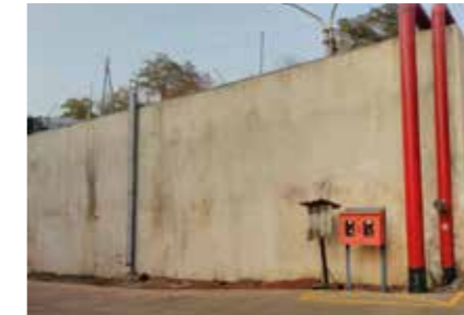
Dedicated water storage tank for fire fighting
