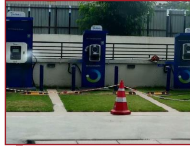
EV charging infra for employees
