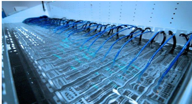
DATA Centre Cooling
