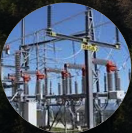
Air Insulated Switchgear (Instrument transformers, Disconnectors, Circuit Breakers)
