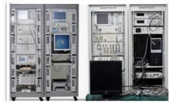
ATE ATS - Facility
