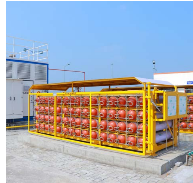
CNG Station (Cascade for Storage)
