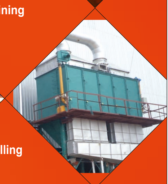
Air Pollution Control System
