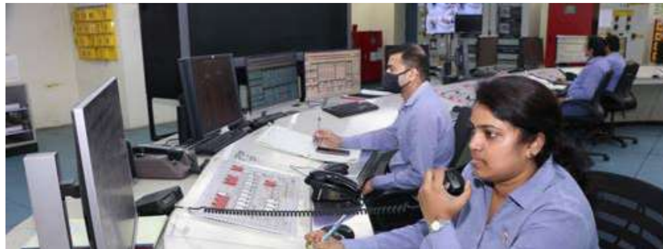
Power plant control room
