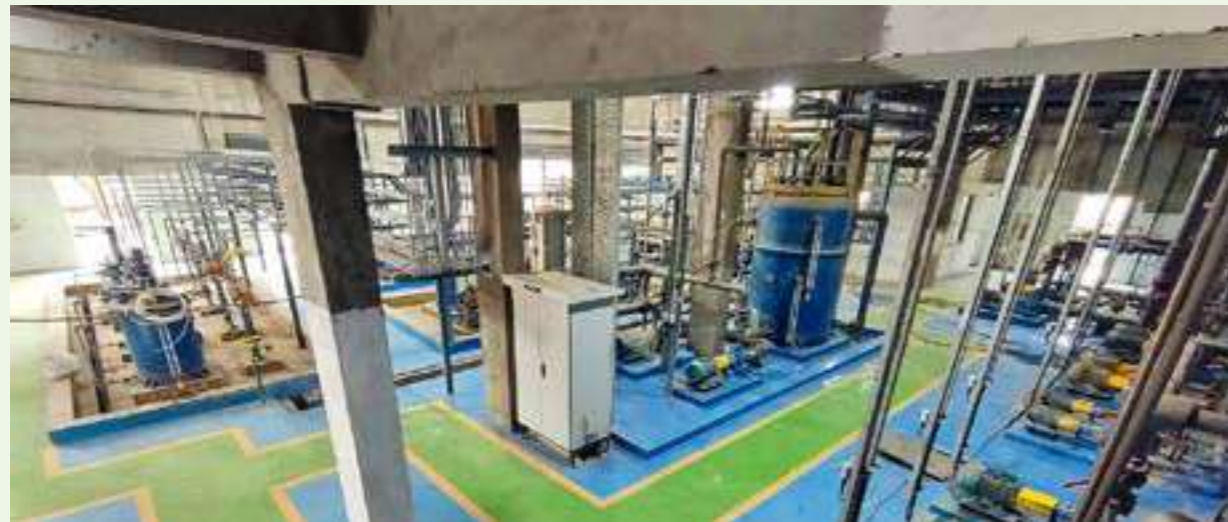
TWRU Pump house
