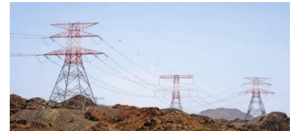
Transmission Lines, Fujirah, Dhaid
