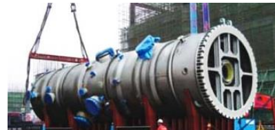
Coal Gasifier for China
