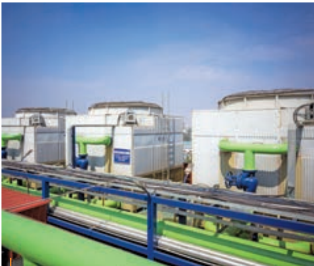
Cooling towers at Biocon Park, Bangalore
