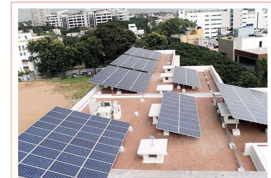
Installed 1MW Solar Power Panels through PPA with Amplus Solar, the installed capacity now stands at 1.7MW
