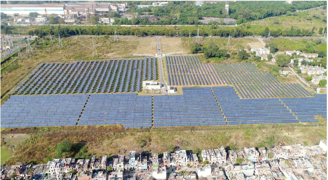
5 MW in-house solar PV installation at BHEL Haridwar for captive power generation
