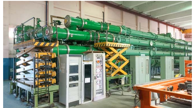
400kV Gas Insulated Switchgear (GIS) bay at Chamera HEP indigenously developed by BHEL under the Aatmanirbhar Bharat initiative
