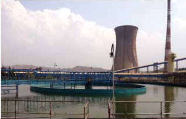
|||||| KPCL Ash Water Treatment Plant, Bellary, Karnataka
