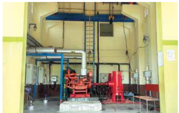
|||||| Gulguli Pumping Station, Cuttack, Odisha
