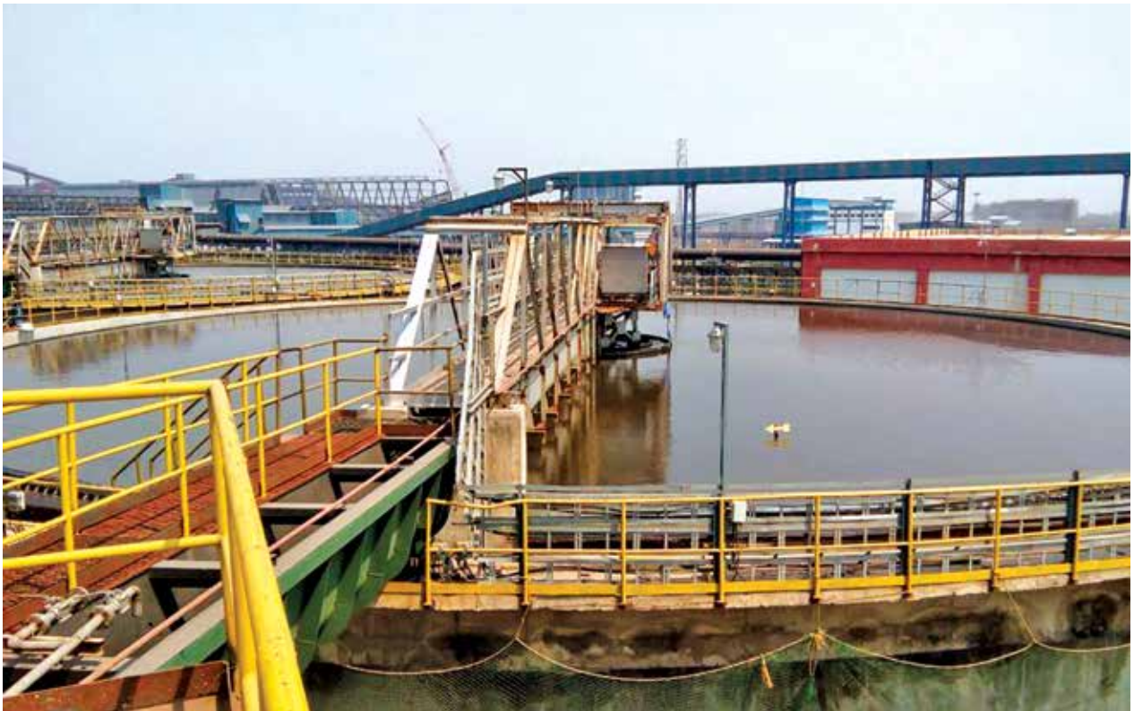
||||| Zero Liquid Discharge Plant For Bank Note Paper Mill, Mysore
