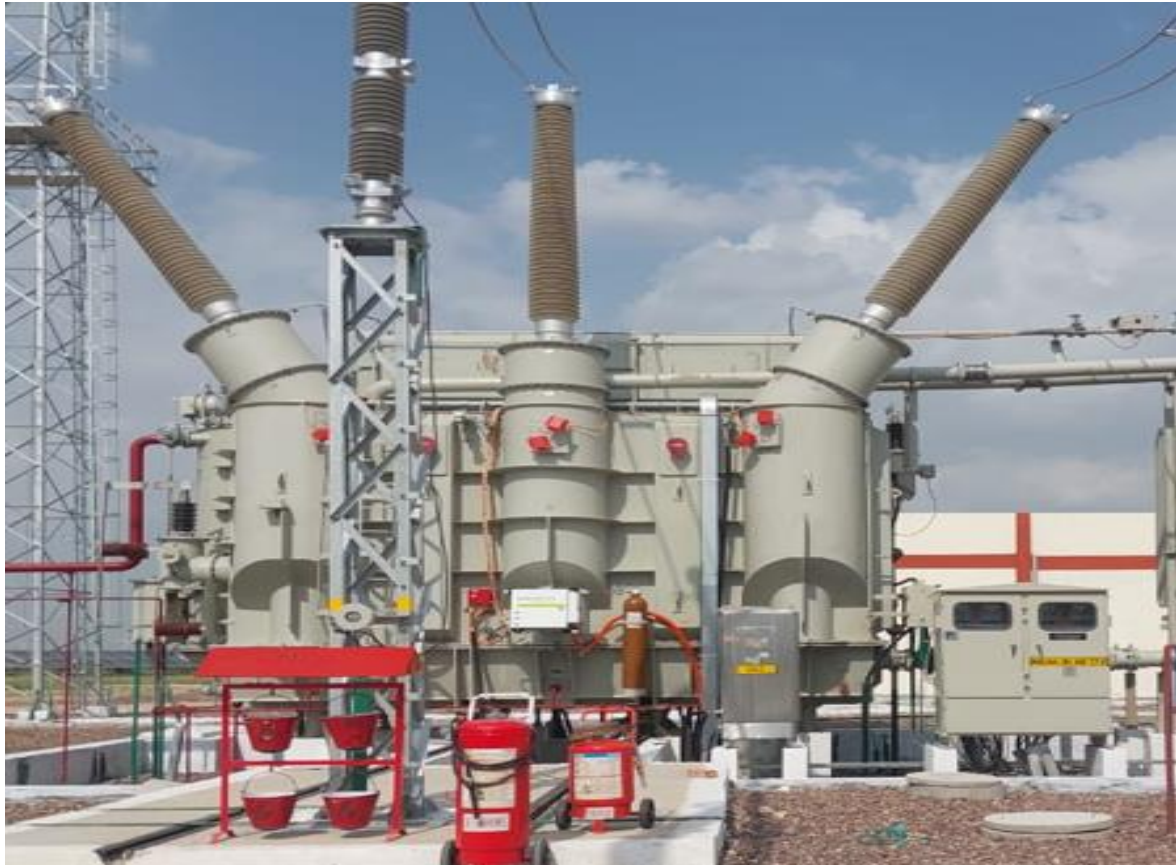
400kV, 375MW substation in Jaisalmer, Rajasthan
