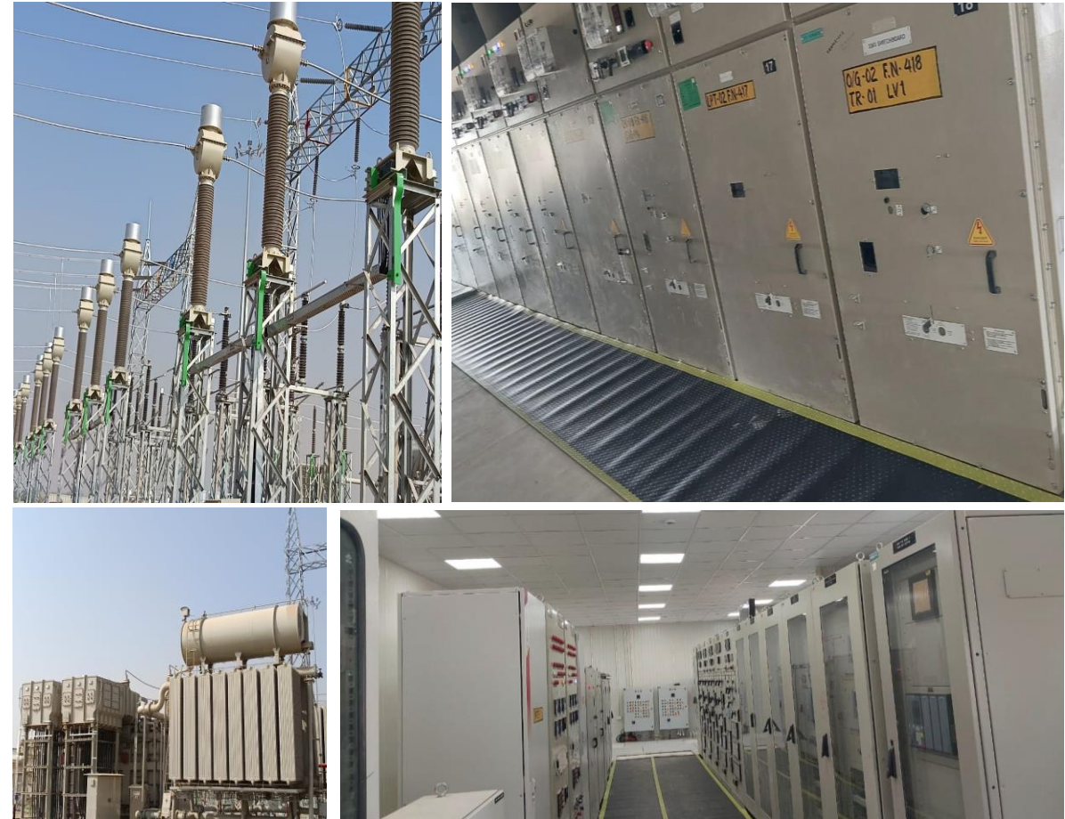
500MW Solar integration s/s in Fatehgarh, Bhimsar and 600MW s/s for NHPC in Baiya, Rajasthan
