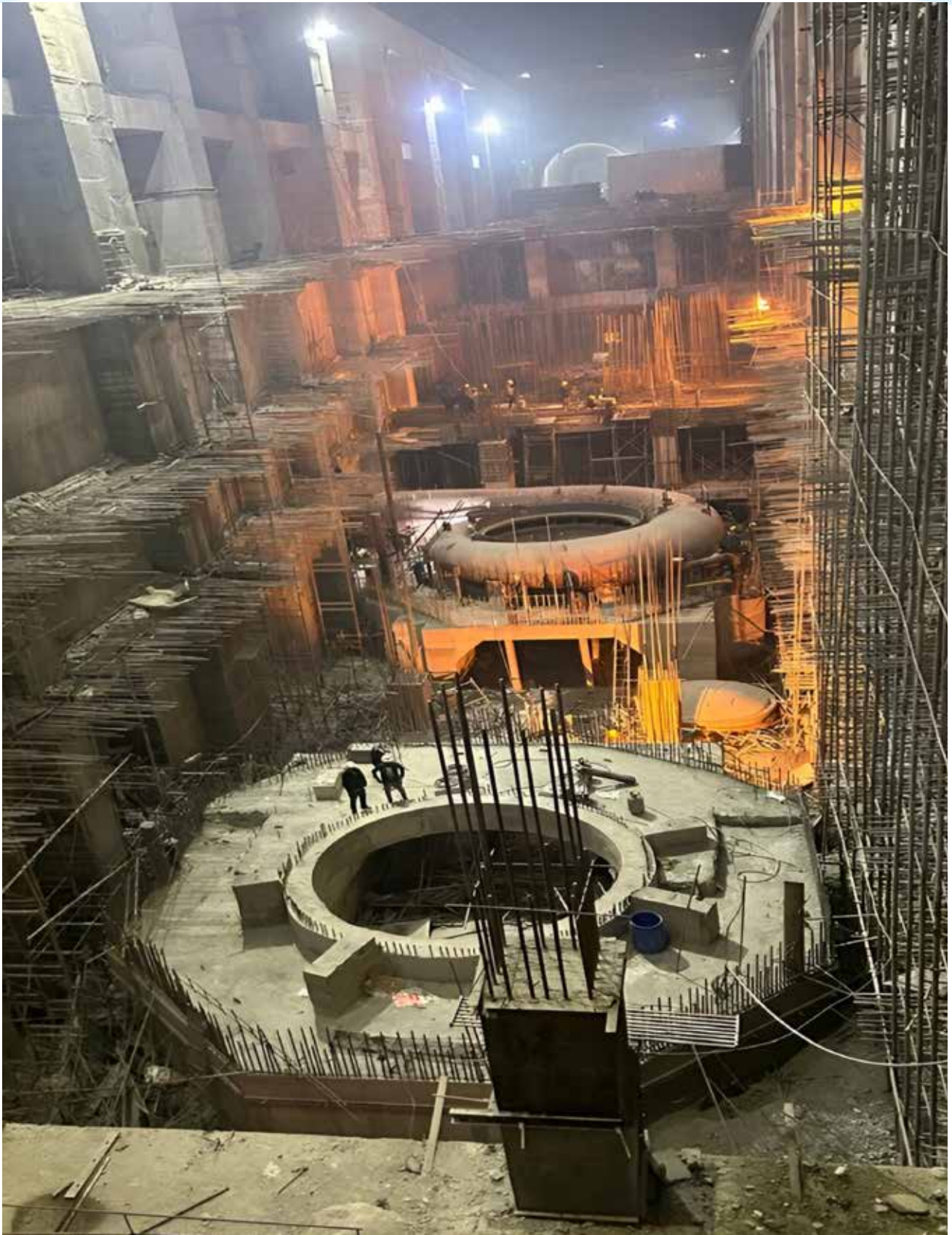
ELECTROMECHANICAL WORKS AT POWER HOUSE – 1000 MW PAKALDUL (UT OF J&K)
