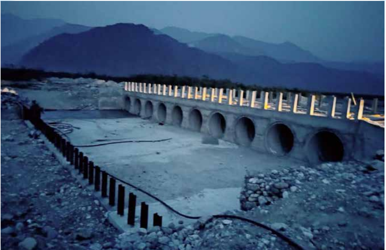
CONSTRUCTION OF APPROACH / HAULAGE ROAD AT RIGHT BANK - DIBANG MULTIPURPOSE PROJECT (ARUNACHAL PRADESH)
