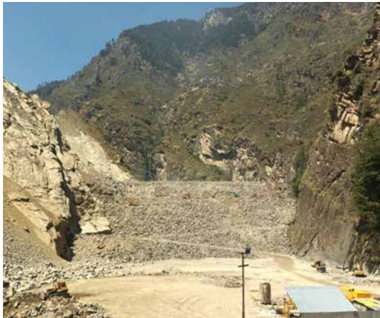
FILLING OF 167 M HIGH CONCRETE FACE ROCK FILL DAM – 1000 MW PAKALDUL (UT OF J&K)
