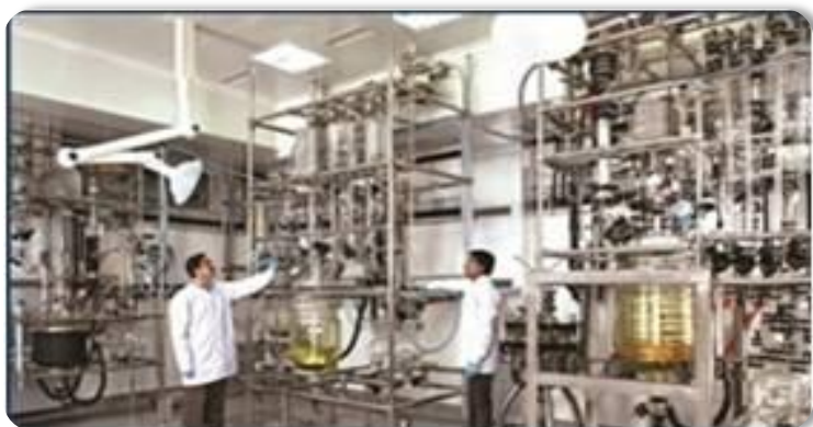
R&D, Contract, cGMP Kilo Lab - Pune
