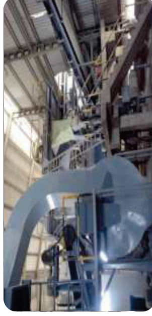
Unit 2– Granulation Plant
