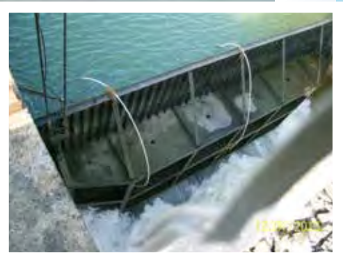
Closer view of one of the new gates in operation
