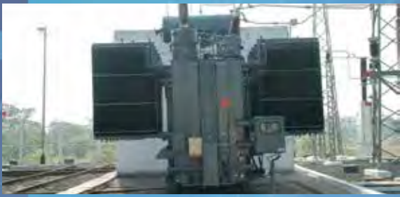
132/27.5KV Power Transformer (rating 21.6/30.24MVA) being erected for Railway Traction Sub Station
