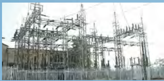
220KV/132KV & 110KV Traction Substation for Railways feeding to 25KV traction
