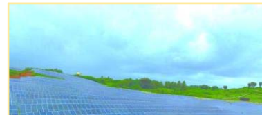
Electricity Department Daman & Diu | 6MW
