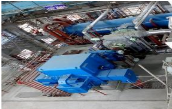
Steam Turbine Generator (STG)
