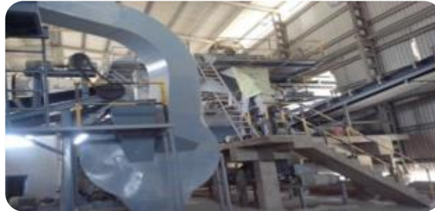
Unit 2– Granulation Plant
