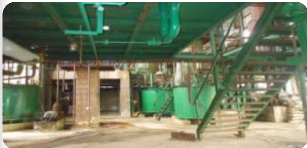
Sulphuric Acid Plant
