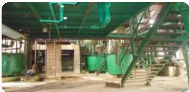
Sulphuric Acid Plant
