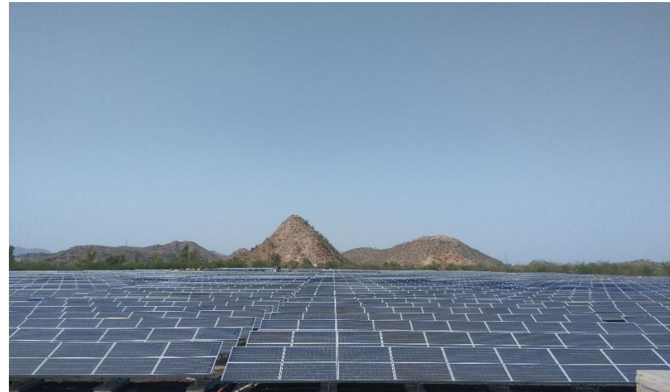
Hindustan Zinc Limited solar panels
