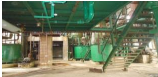
Sulphuric Acid Plant
